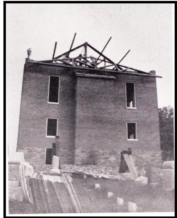
Dismantling of the Third Church, 1914. The building was razed without charge by members of the congregation.
